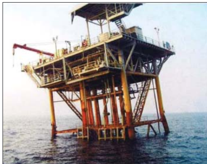
A hurricane probably caused the foundation of this platform to fail (Fig. 3). Photo from US Minerals Management Service.
